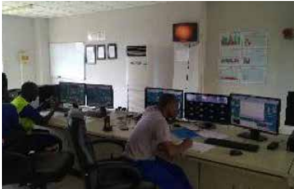
Factory's control room
